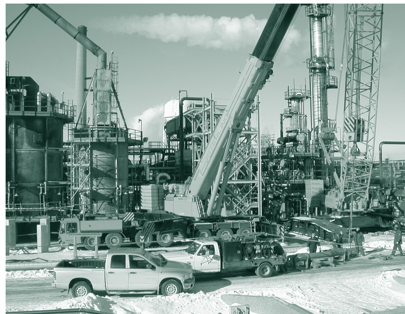
Planned shutdowns are opportune times to add new technology for environmental improvements. This photograph shows a new high efficiency, low-NOx heater being installed on a reformer unit at the Shell refinery in 2005.
